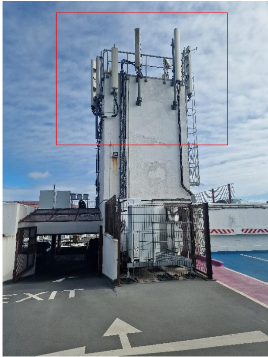
Sand Street Car Park – 40.89% of ICNIRP guidelines
